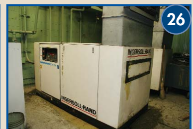
INGERSOLL RAND 100 HP AIR COMPRESSOR
